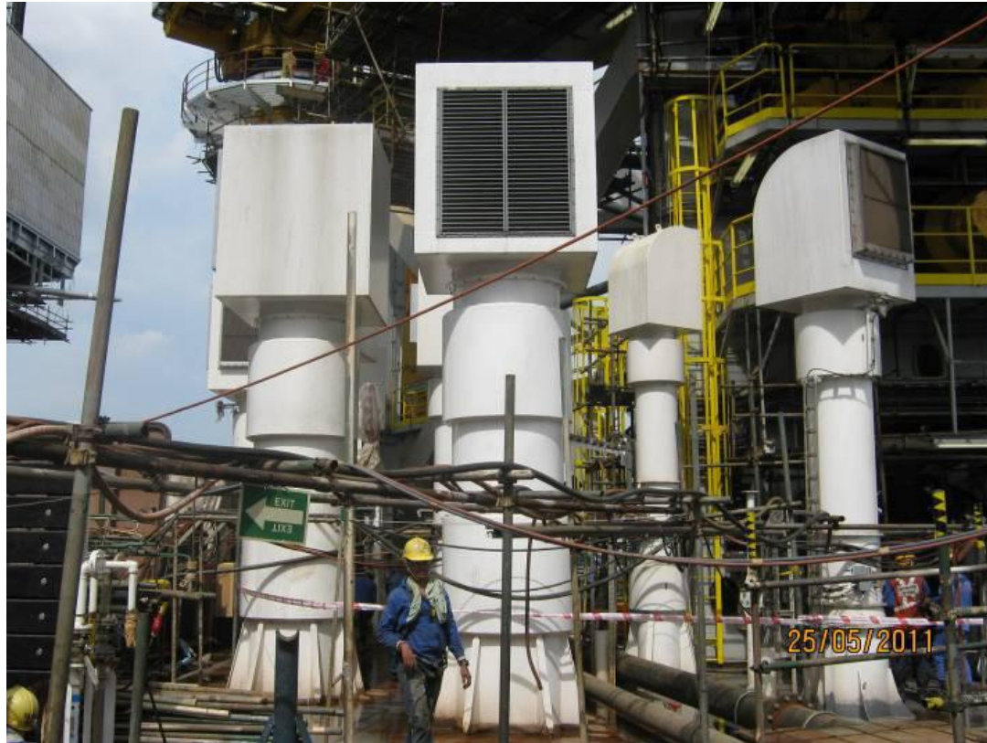
Air exhaust and inlet on main deck injection fans - exhaust line
